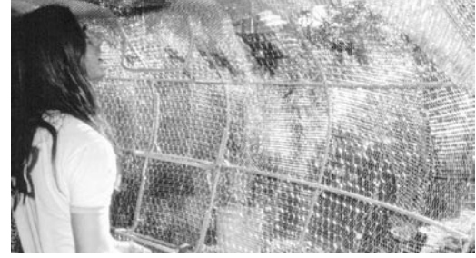
A lath and chicken-wire matrix are tied tightly to the rebar frame.
